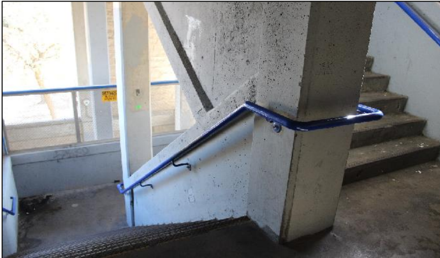
Improving visibility on the stairs was identified as a way to improve safety while transferring.
