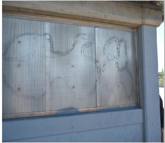
Image 26 (Incomplete graffiti removal)
