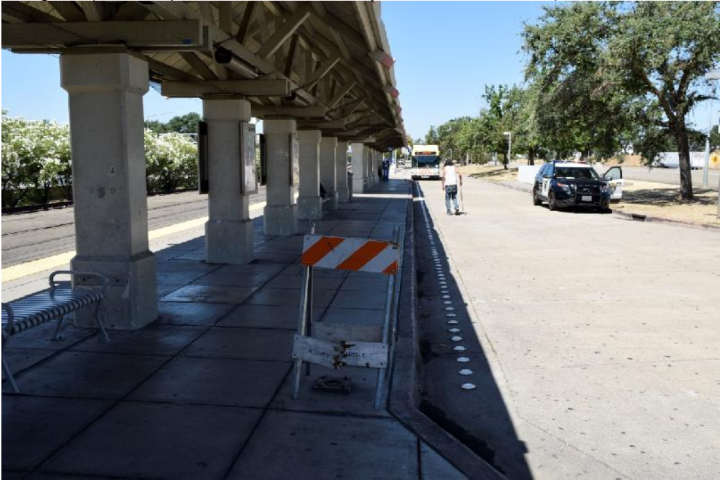
Image 4 (broken pole base covered by broken barricade)
