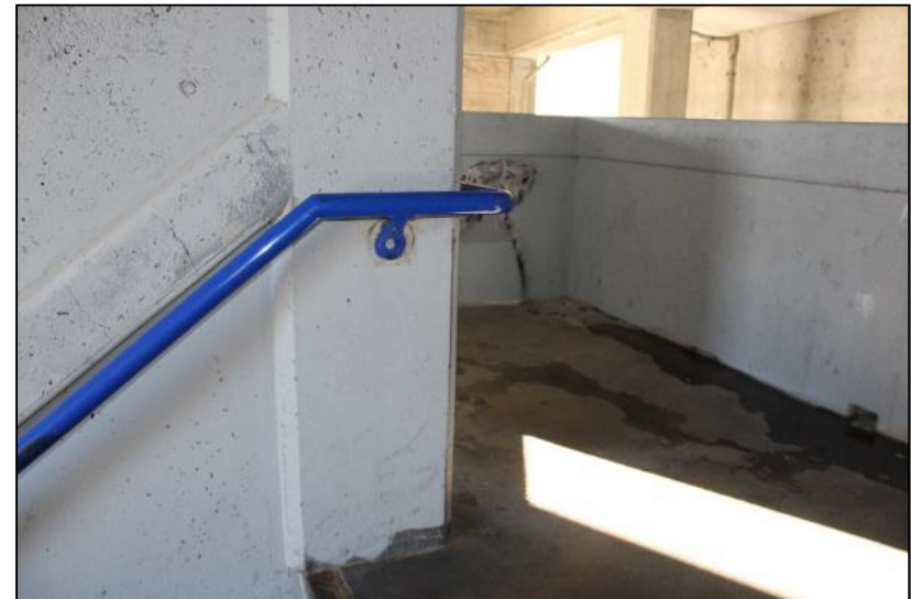
Sharp corners block visibility on the stairs.
