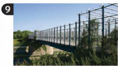
Enhanced Protective Railing
