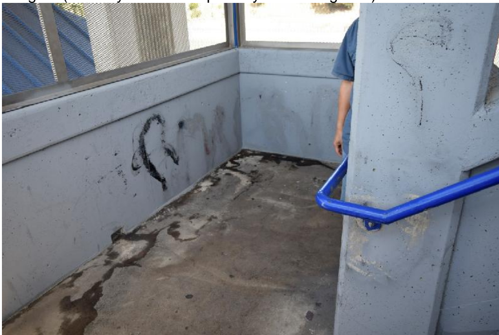
Image 7 (stairway "toilet" and partially removed graffiti)
