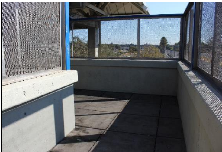
Sharp corners hide the stair access point. Concrete and shade structures create dark areas and prevent natural light from entering the space.
