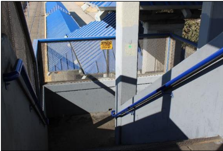
Shadows, sharp corners, and concrete columns create hiding spaces and contribute to safety concerns.
