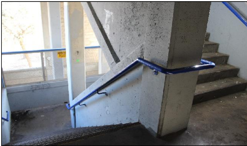
Steep stairwells, sharp corners, and low visibility contribute to an unsafe and unpleasant transfer environment.
